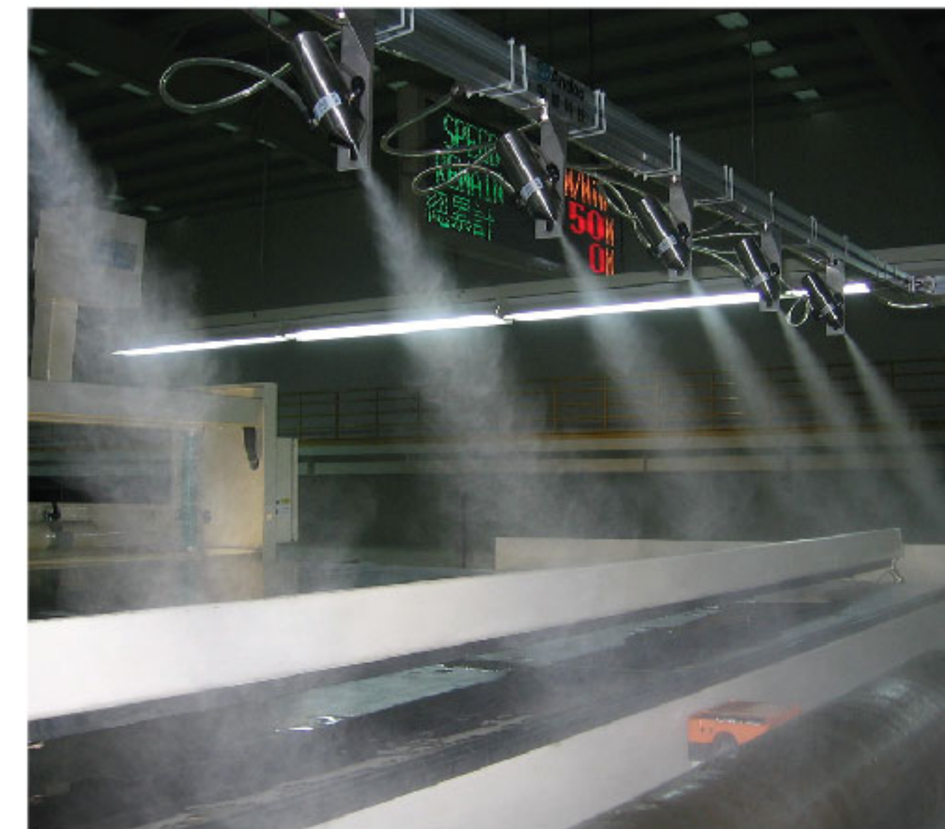
喷雾加湿 Spraying humidification
